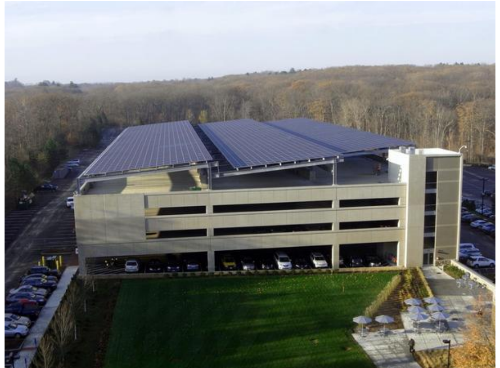
685-kilowatt installation at Staples headquarters in Framingham
